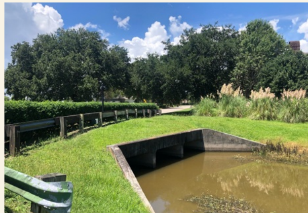
Current condition of the Delacroix Canal.
